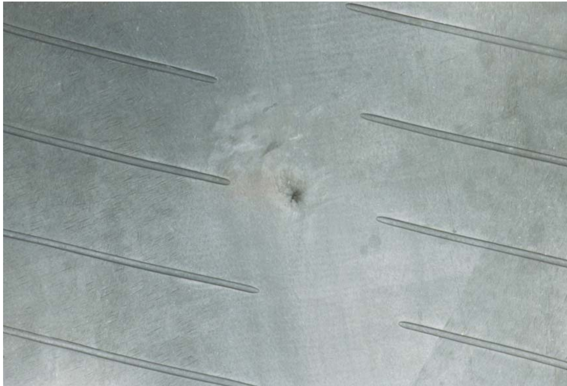
Figure 6 - Arcing hole on Position 6
